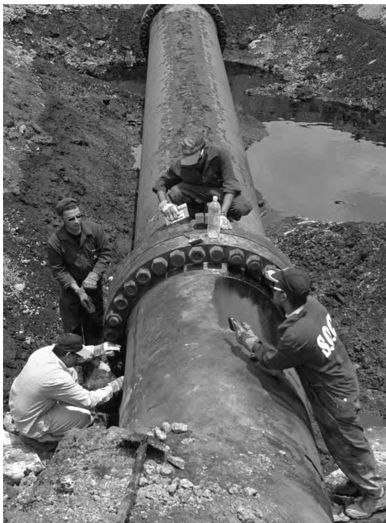
A damaged oil pipeline near Basra, Iraq, with the world's third largest oil reserves, has to struggle to keep oil exports flowing.
